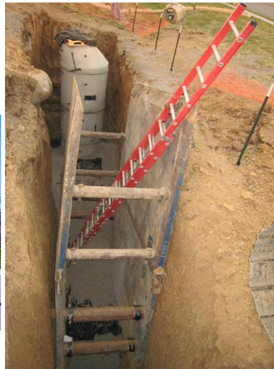
Figure 10-14 Trench boxes and many other tools come from shoring services type companies
